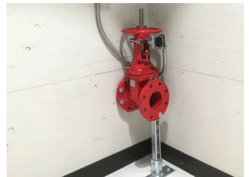
New OS&Y and water flow valves were mounted at each fire alarm station as part of the upgrades for the Fire Alarm Lab.
